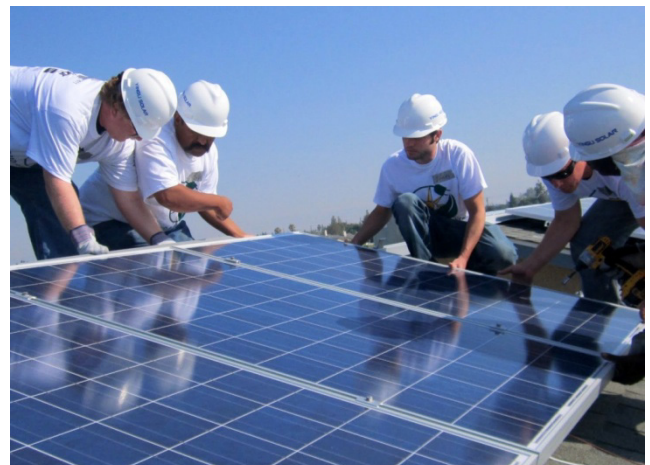
Grid Alternatives volunteers set down solar modules on a low-income family's rooftop in Fresno, CA
